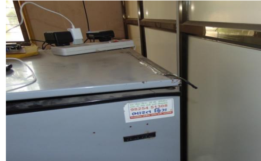
Fig.III.V Room temperature sensor
