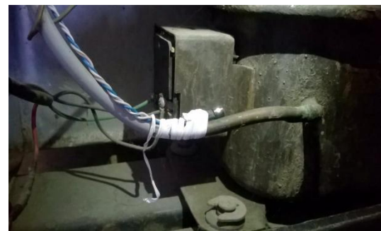
Fig.III.VII Compressor input temperature sensor
