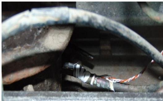
Fig.III.VI Compressor output temperature sensor
