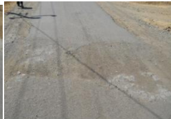
fig.5 Spalling of Agg.
