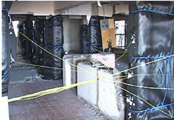
Fig.3.3.Columns fully loaded with explosives and hooked up to blasting caps and fuses.
