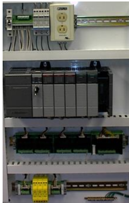
Fig. 5 A rack type PLC
