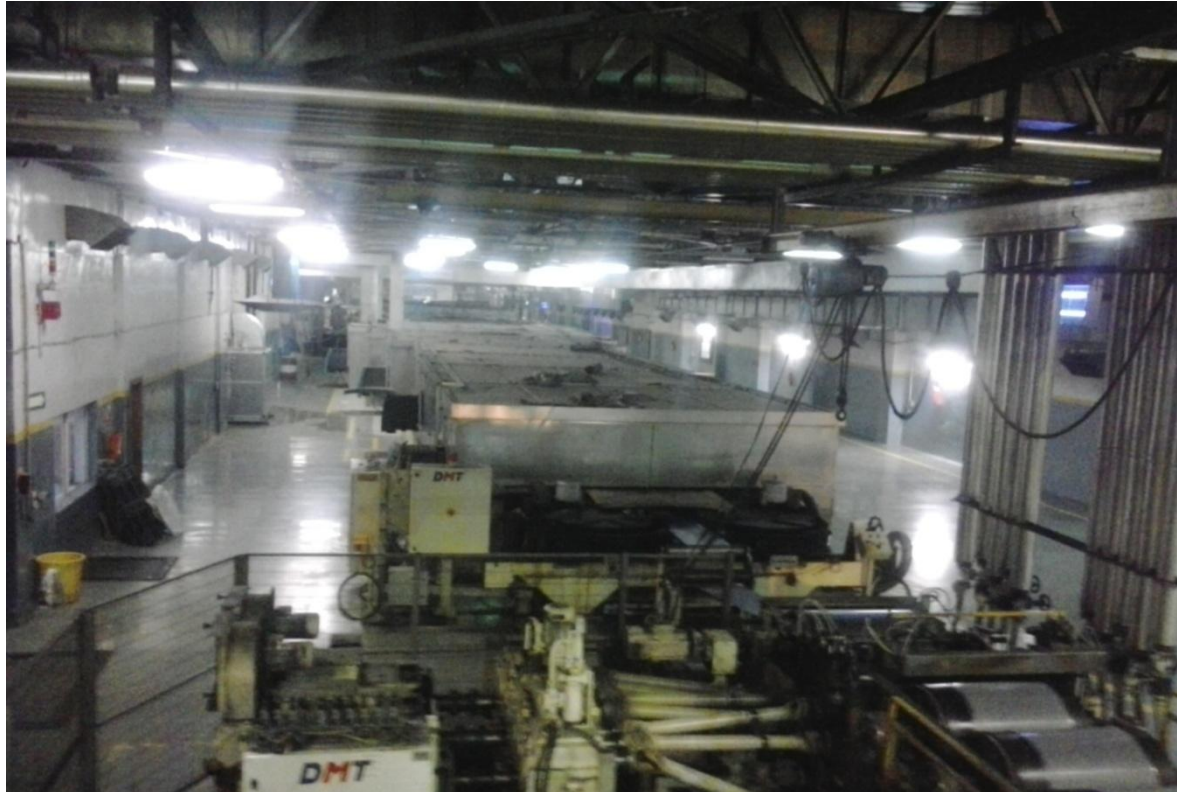
Fig. 4 Transverse direction orientation (TDO) before modification.
