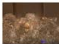
Figure 2: Corrosion on tube
